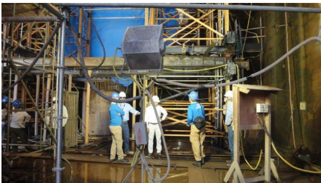
Photo 49: Inside Right Bank Power House - safety hazards.
