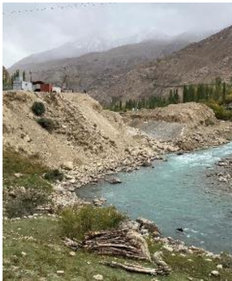
Photo 94: Unstable riverbank immediately downstream of the intake
