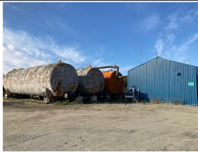
Photo 26: Insulated freshwater tanks
