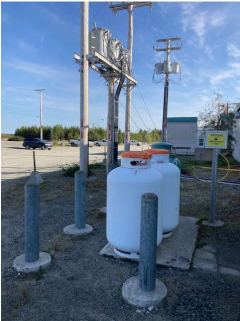
Photo 37: Safety barriers around gas tanks
