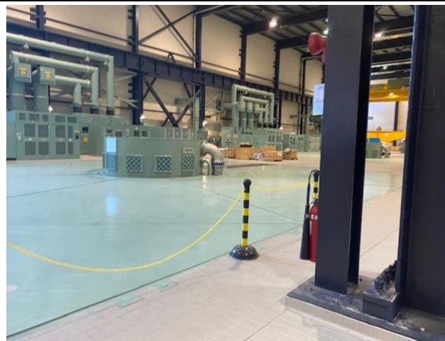
Photo 5: Eastmain-1a powerhouse interior
