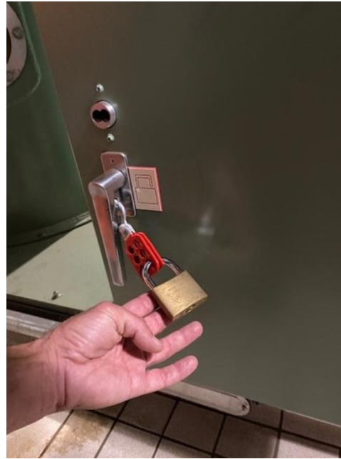
Photo 8: Equipment with personal safety lock
