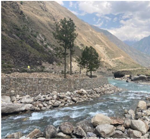
Photo 46: Confluence Chuwa with Karnali, with island belonging to temple protected with gabions
