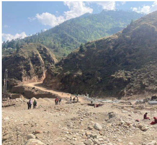
Photo 40: Gravel banks at mouth of Chuwa, laydown area for distribution line poles, women crushing stones for aggregates
