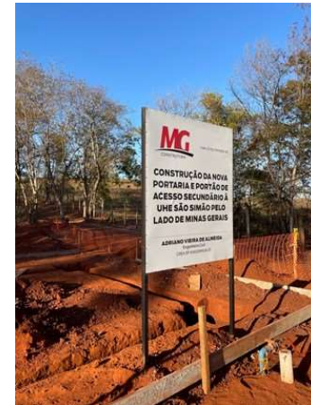
Photo 35: Construction of new gate to access São Simão HPP: activity being implemented by a third party under SPIC's supervision
