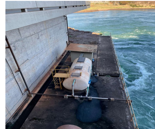
Photo 17: External Sewage Treatment Station adjacent to the powerhouse
