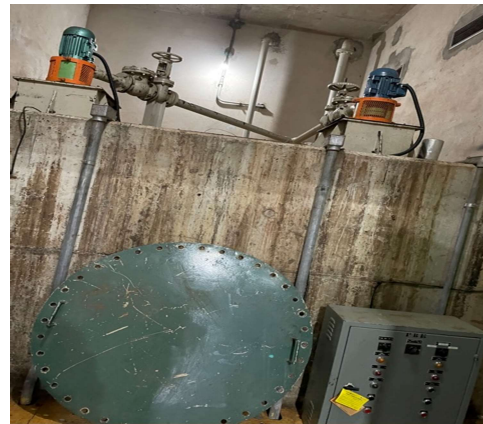
Photo 16: Internal Sewage Treatment Station inside the powerhouse
