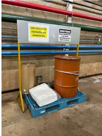
Photo 7: Environmental Emergency Kit Station (one of many) inside the powerhouse
