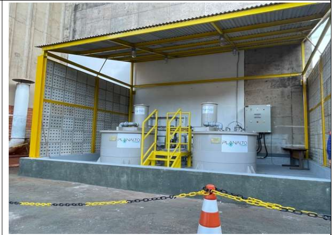
Photo 20: Equipment that prepares and injects chlorine solution to combat to the Golden mussel
