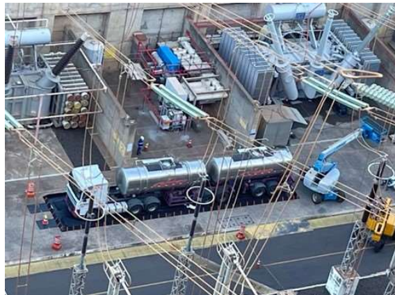
Photo 15: Truck used for the transformer oil change operation completely inside secondary containment equipment developed by SPC Brazil
