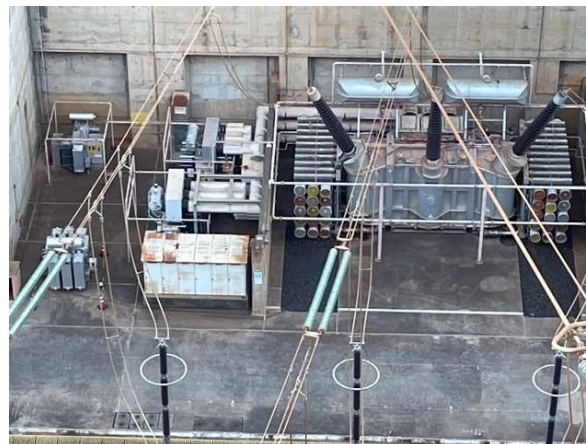
Photo 13: Transformer installed over a containment structure
