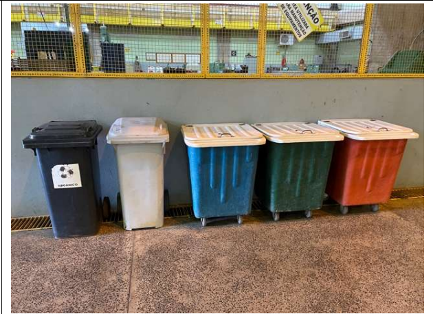
Photo 8: Waste separation station inside the powerhouse
