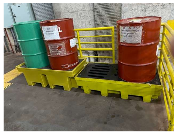
Photo 12: Secondary containment equipment for oil leakage and spill inside the powerhouse
