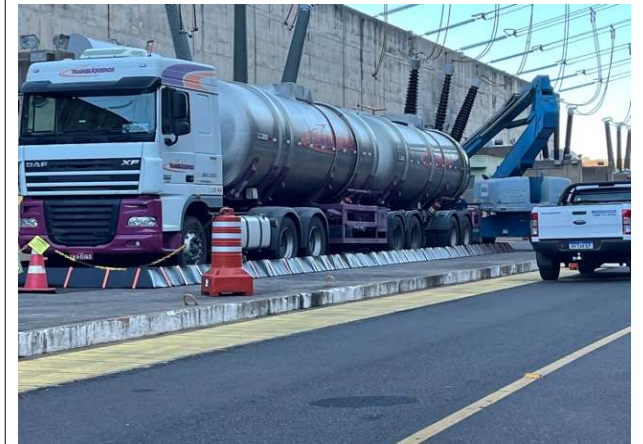
Photo 14: Truck used for the transformer oil change operation completely inside secondary containment equipment developed by SPC Brazil
