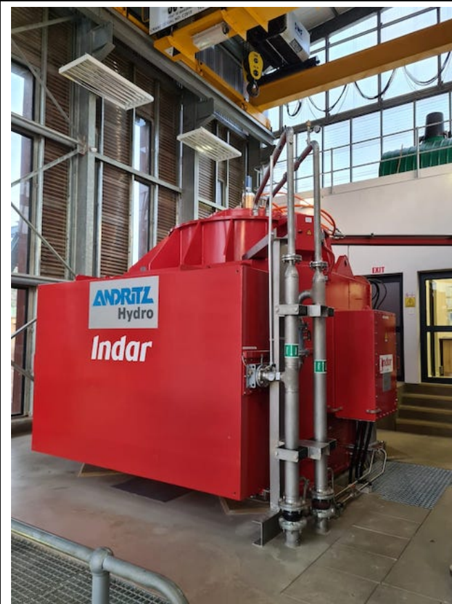
Photo 19: Generator with door to control room
