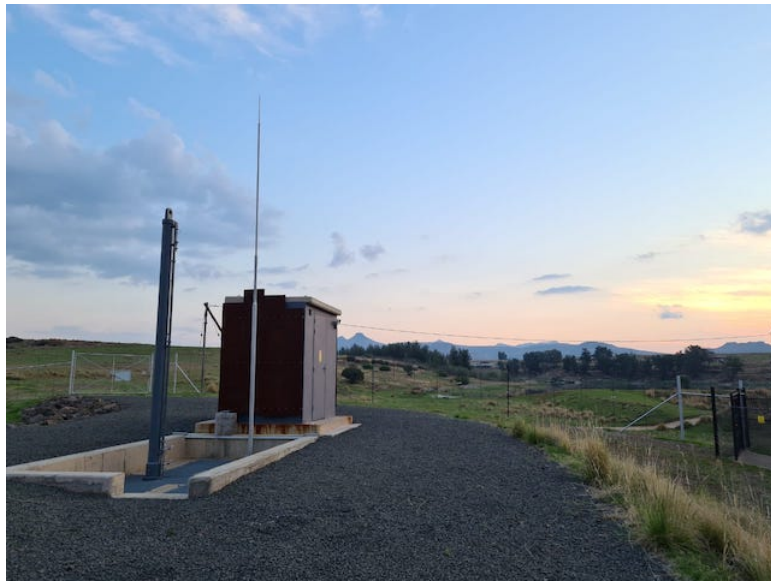
Photo 8: Intake gate controls, with Boston A farm dam in background
