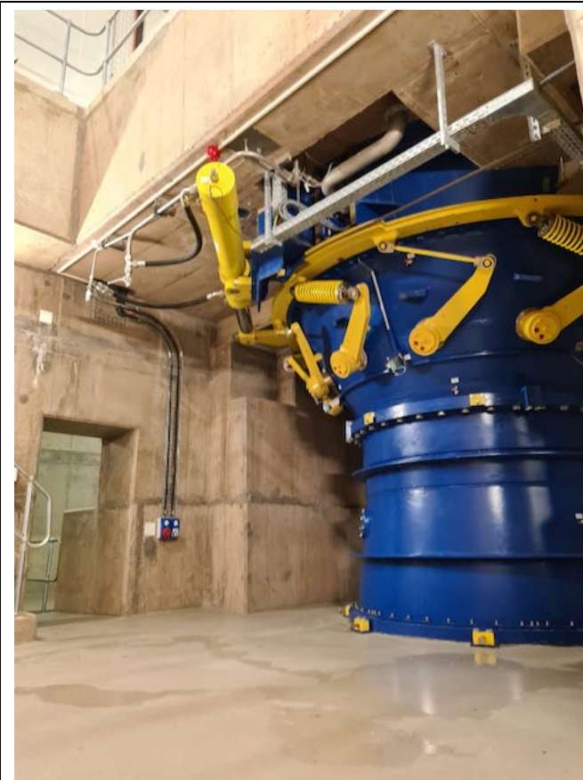
Photo 16: Guide vane controls
