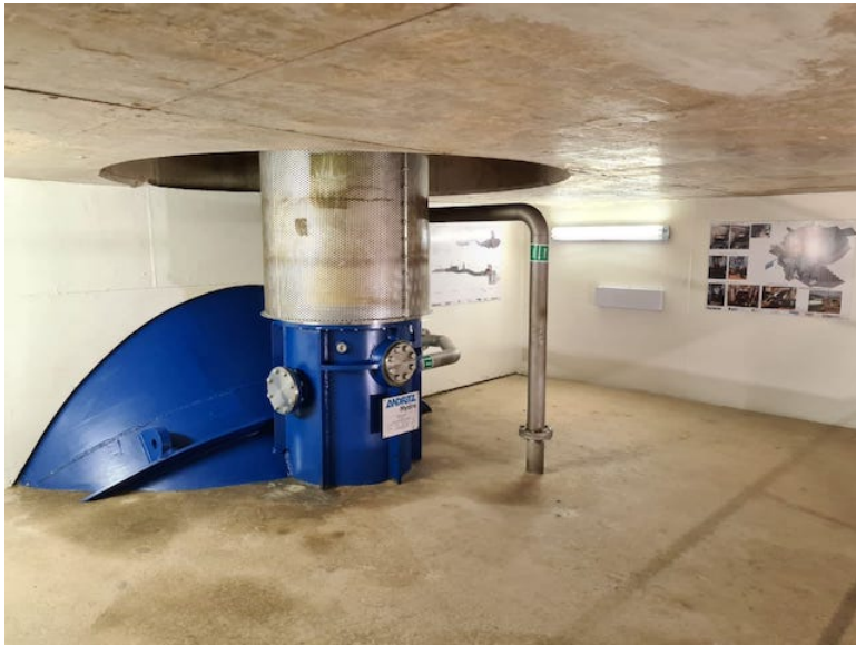
Photo 12: Penstock entering powerhouse
