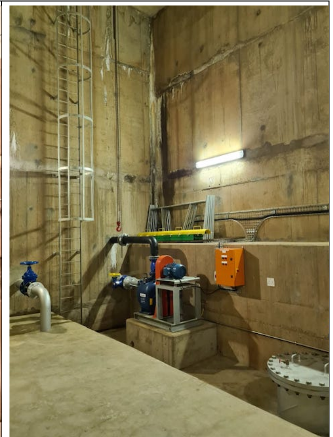
Photo 18: Sump pump and escape hatch ladder
