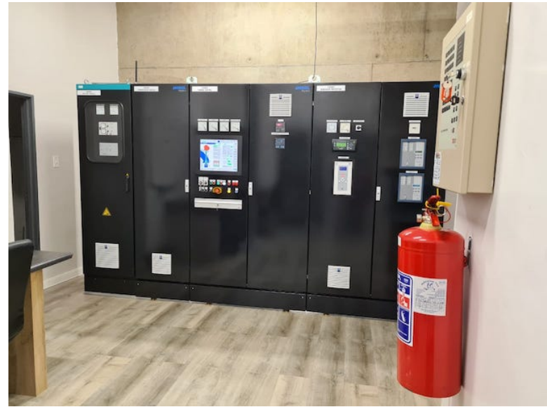
Photo 13: Panels in control room
