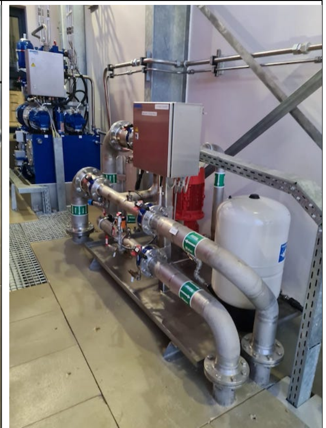
Photo 21: Cooling system on ground floor
