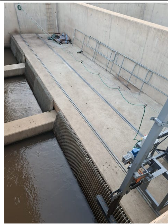
Photo 5: Fine trashrack with cleaning machine
