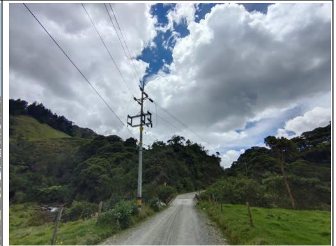
Photo 9: Existing power lines 2
