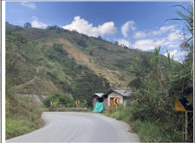
Photo 36: Storage sheds above future powerhouse, with unstable slopes above 25AN road
