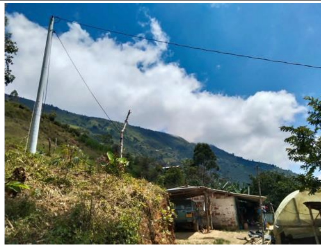
Photo 8: Existing power lines 1
