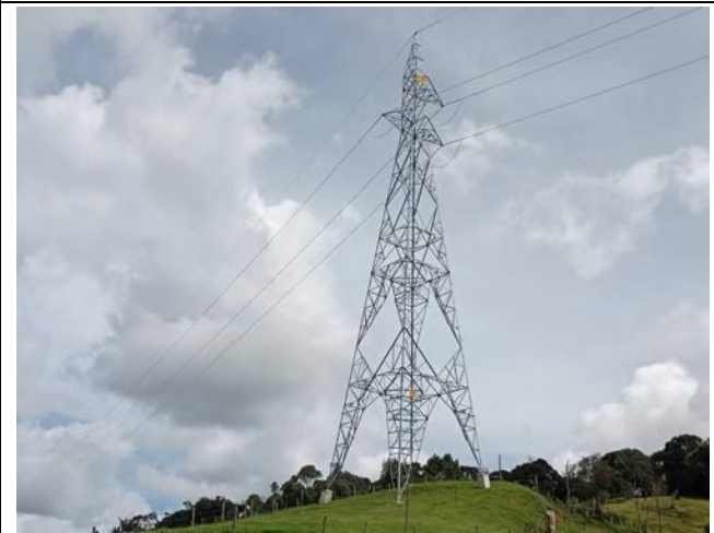
Photo 10: Existing power lines 3
