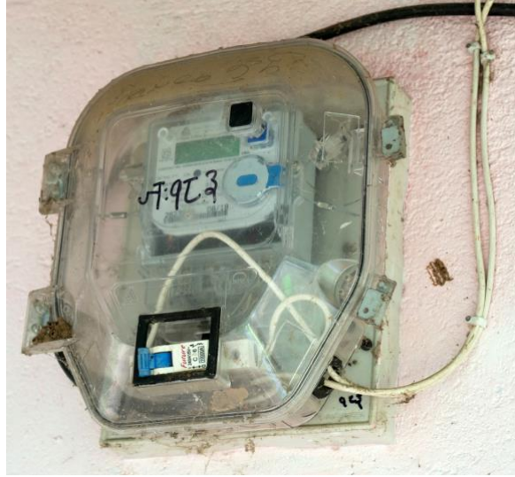
Photo 32: Electricity-connection box at the resettlement house.
