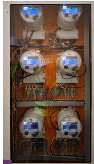
Photo 53: Automatic record-keeping on generation at the substation.
