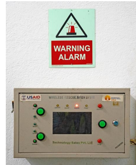
Photo 30: The emergency alarm can be triggered remotely by calling this device, located inside the powerhouse.
