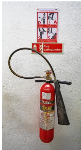
Photo 10: Fire extinguishers are found in several key locations around the plant.
